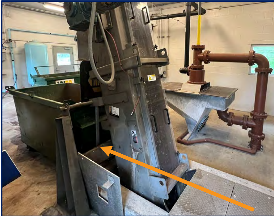
Screens remove large debris before further treatment
